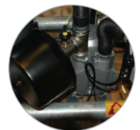
Inlet blower filters
