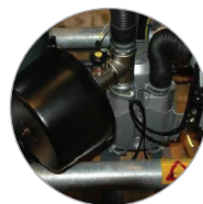
Blower inlet filter
