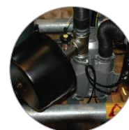
Inlet blower filters
