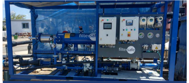
RO Membrane Protection Project
