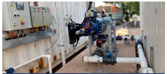
RO Membrane Protection Project
